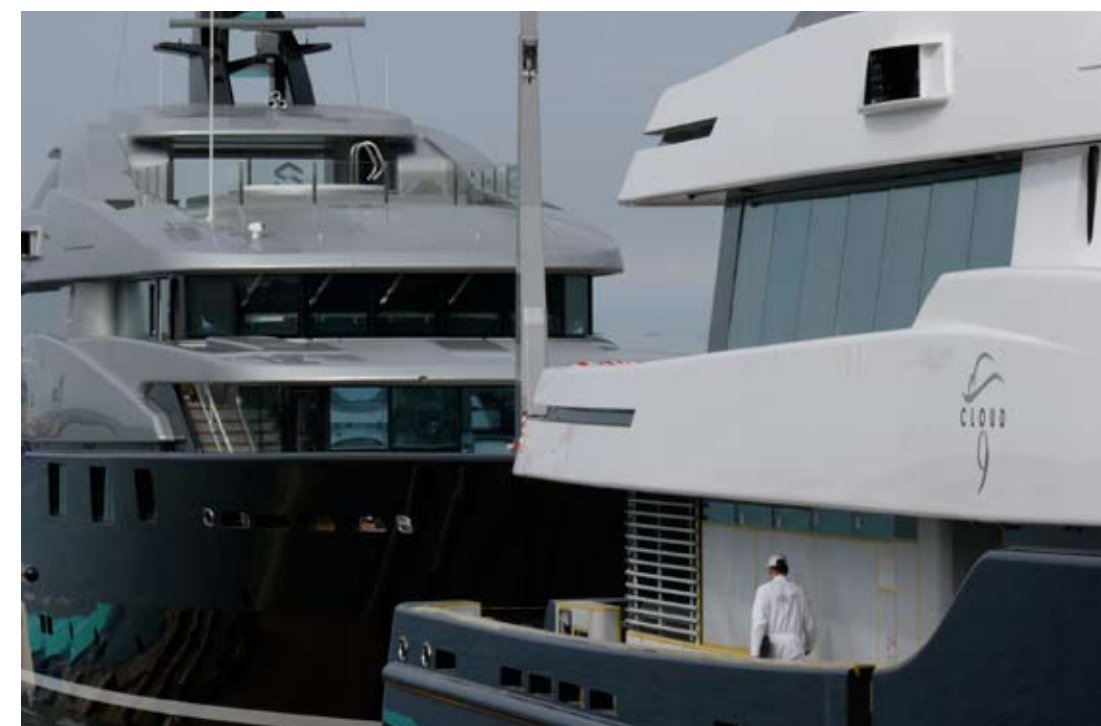
Above & Far Left: ‘Slipstream’ takes shape in one of CMN’s large covered building sheds.
